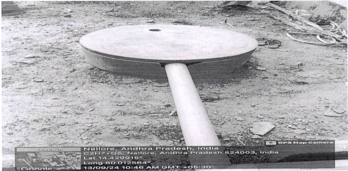
GEO TAGGED PHOTO OF RAIN HARVESTING SYSTEM
