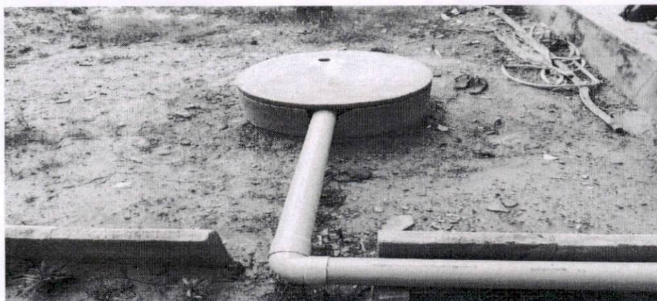
Fig.1: Rain Water Harvesting (RWH) system implemented in the College
