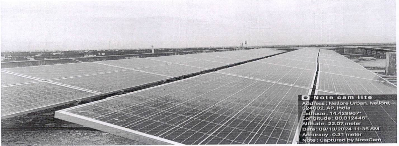
Roof top solar energy panel geotagged photos
